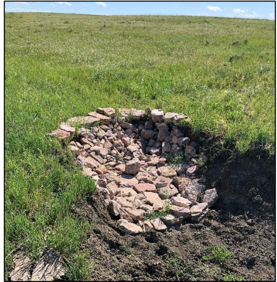
One of the structures the group saw on the first day: a rock run-down structure that helps to stop a head-cut from eroding further.
