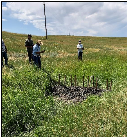
One of the beaver dam analog structures built on the second day. This will help slow water, allowing sediments to deposit and helping to restore riparian area vegetation.
